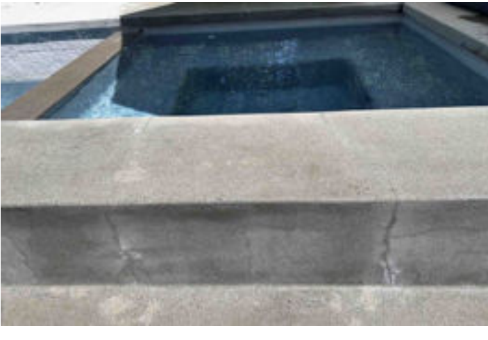
Structural Crack or Not?
